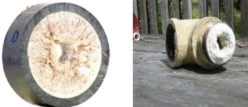
Figure 1: Struvite formed in wastewater pipes (Apex Solutions, 2012; Merrill, 2012)
