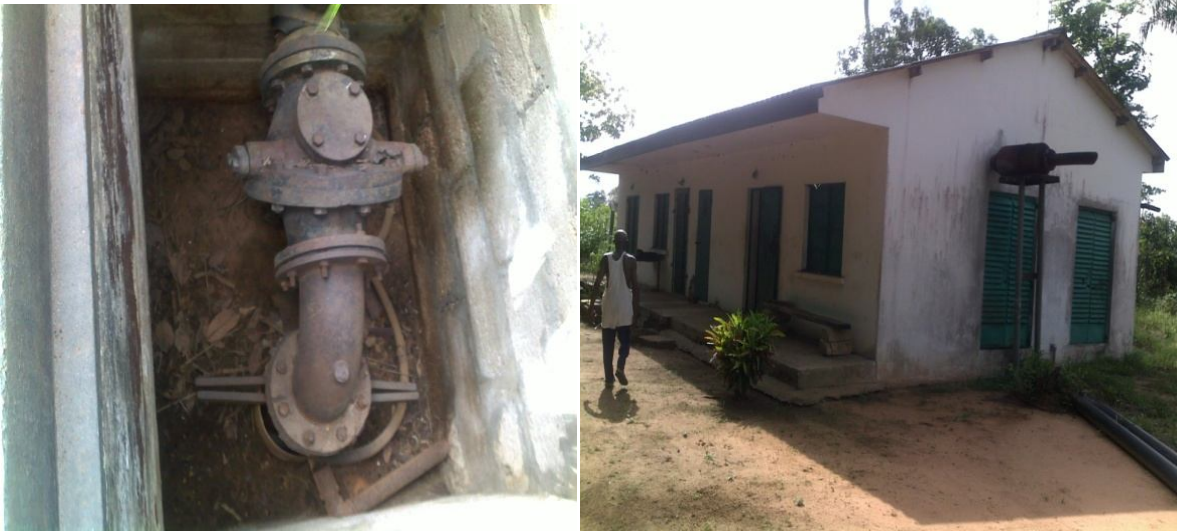
Figure 4: Headwork of Obiaruku Water Scheme
