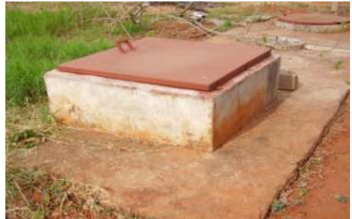
Figure above shows underground Dome Digester
