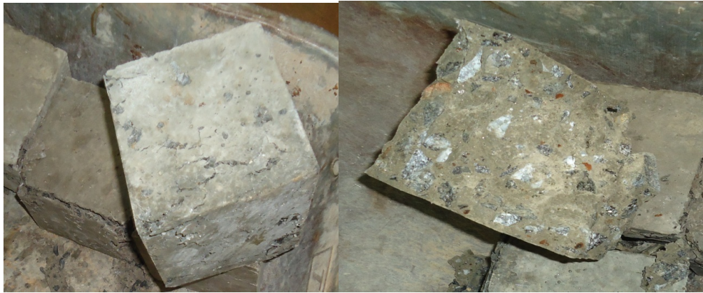
Fig. 5: Failure of PKS aggregates
