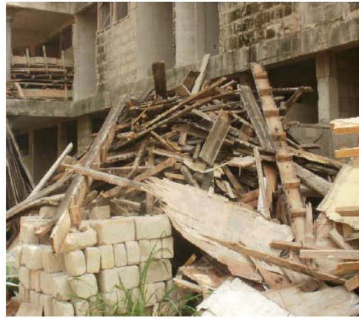
b) Dismantled formwork left on site
