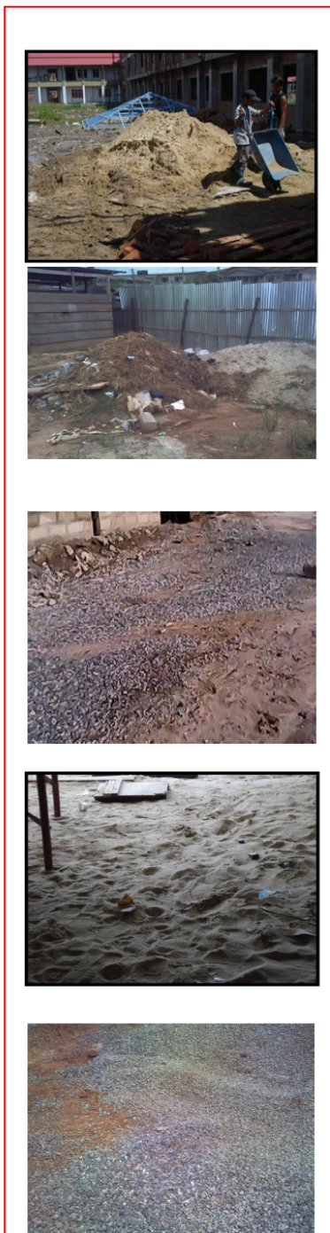
Fig. 8a: Ways in which Materials for Concrete Production are Wasted on Site
