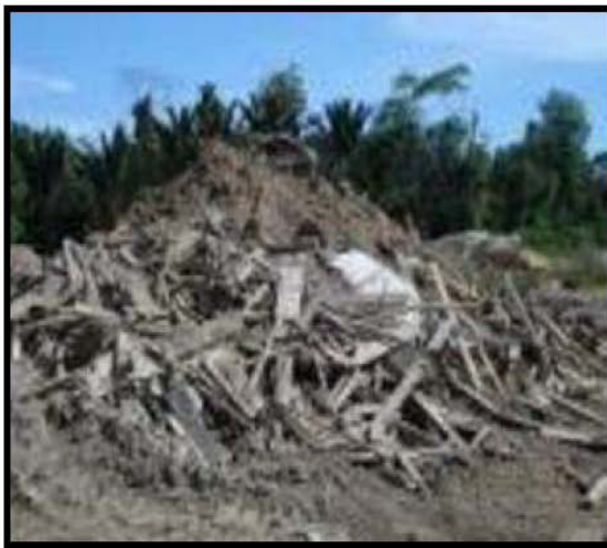
c) Timber pieces left to decay on site
