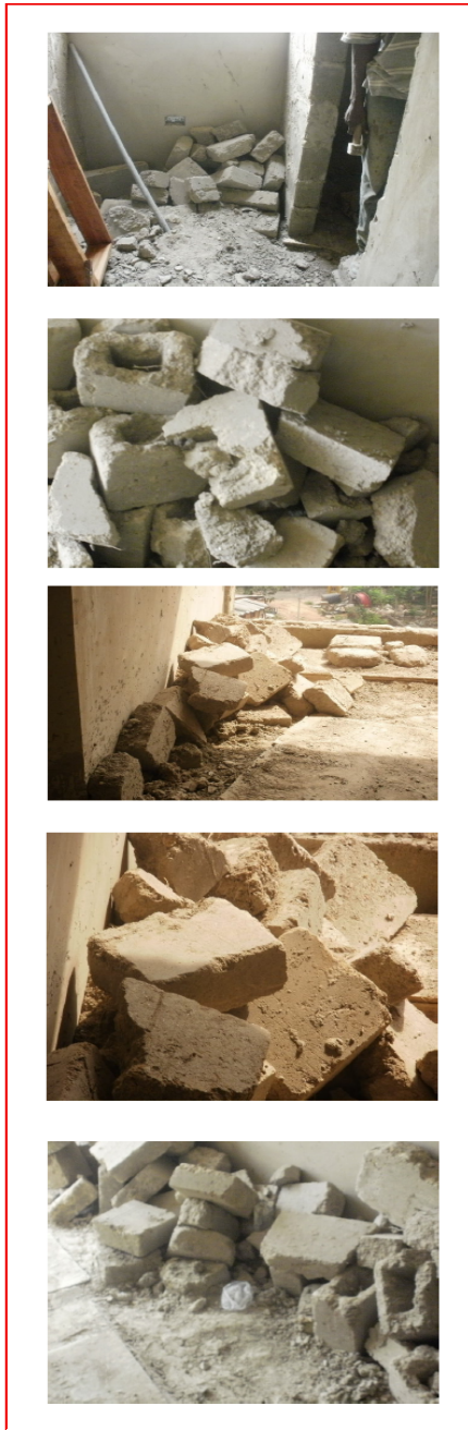
Fig. 9 a: Wastage of Blocks on Construction Sites
