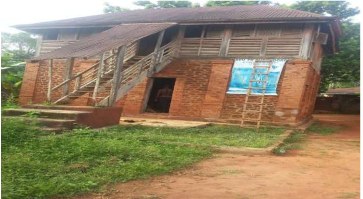
PLATE 2: This building was a residential quarter for a German missionary who died in 1924, constructed with a combination of locally available stone and mud
