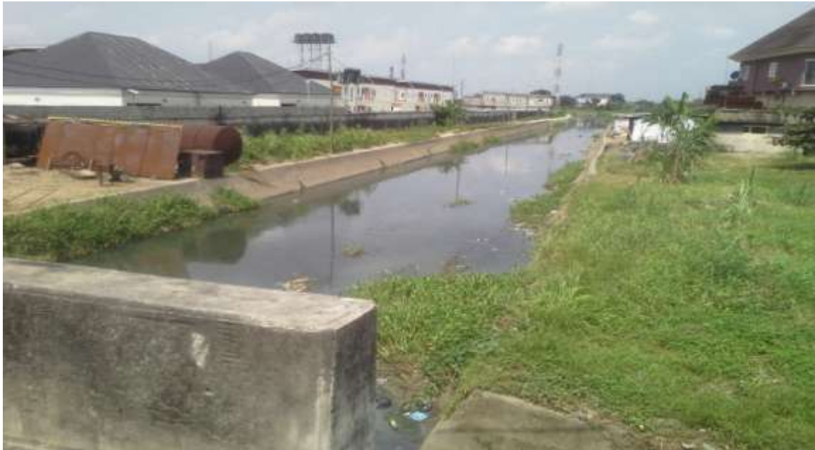
Plate1.7: Showing Culvert Obstruction Of Ntawogba Creek Along Cherubim
