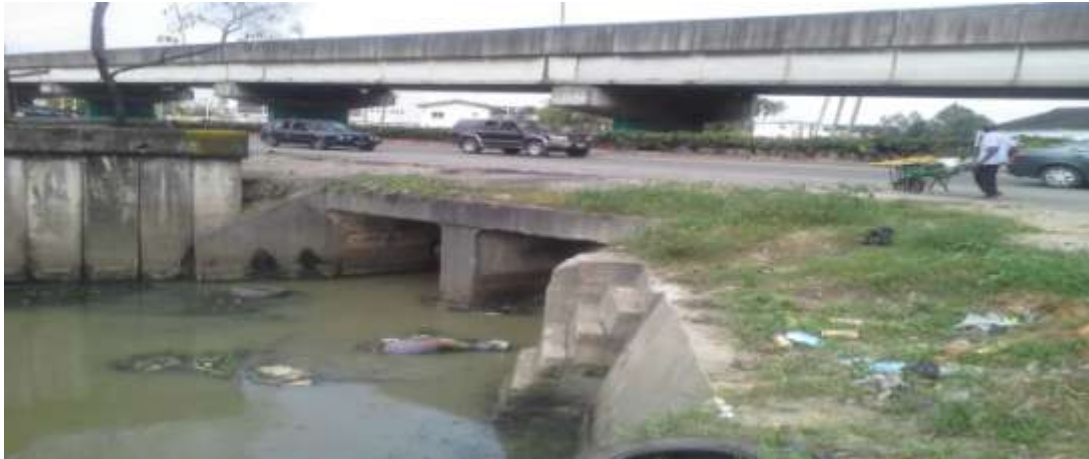
Plate 2.2: Showing Obstruction Of Ntawogba Creek Along Aba Road
