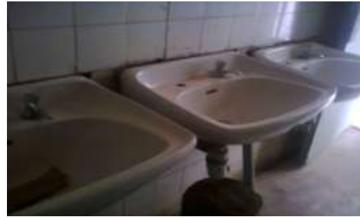
Figure 13: Poorly installed plumbing fixtures
