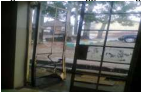
Figure 8: broken door panes
