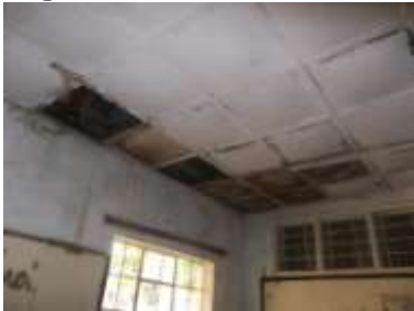
Figure 6: Water logged ceiling
