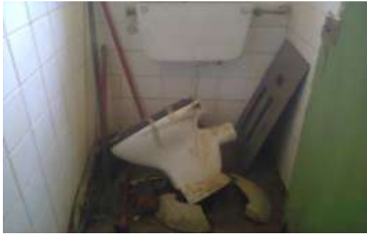
Figure 12: Broken water closets
