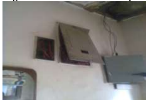
Figure 11: Poorly installed electrical fittings
