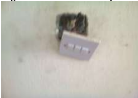
Figure 10: Poorly installed electrical fittings
