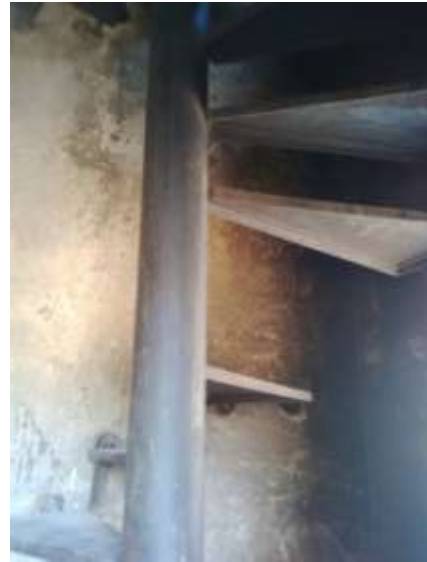
Plate ix: spiral stairs without handrails
