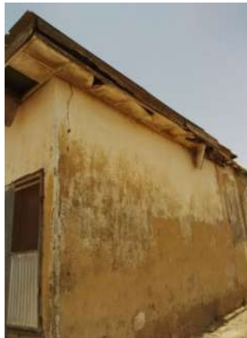
Plate iii: Walls with cracks
