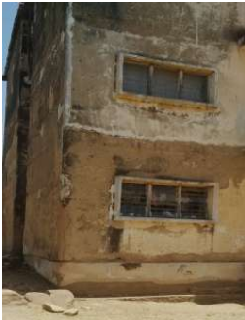
Plate ii: Walls with plaster falling off
