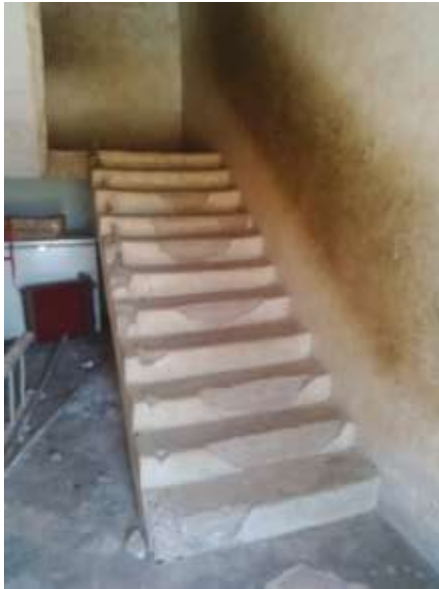
Plate viii: Stair ways without railings
